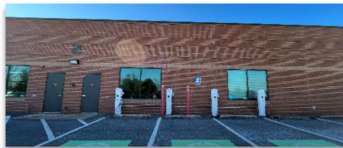
Electric Charging Station
